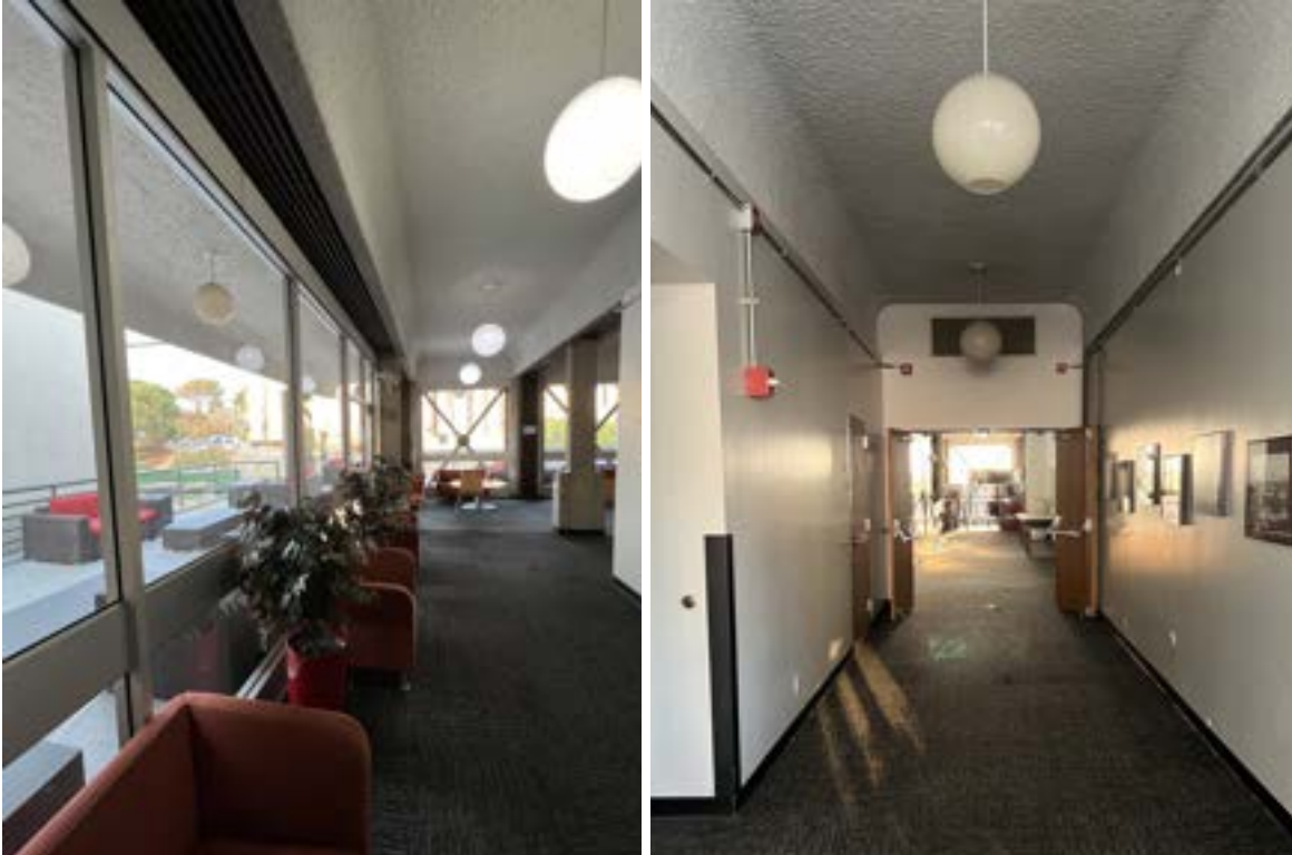
Lighting not working on the third floor of the Old University Union
